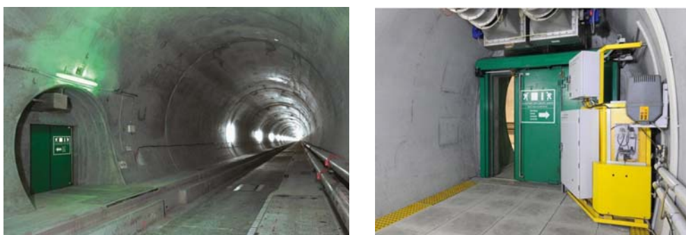
Figure 12. Fire-protection doors in the Gotthard Base Tunnel
